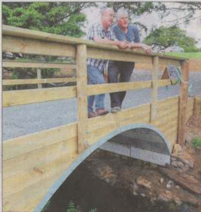
QUICK ASSEMBLY: Steve Swann (left), and Kelly Wright on a 4.6m Clearwater Crossings bridge they have installed on John and Bev Manderson's property at Kauri.
